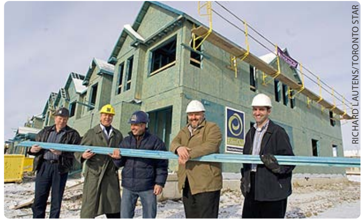
Standing in front of the 22-townhouse development by Eden Oak Homes in Vellore Village in Vaughan, the first development in Ontario to use BluWood for construction are: left to right, Erwin Leonov and Mark Foster of BluWood Canada, Frank Lanza and Bernie Torchia of Eden Oak Homes and Corrado Distefano of Alpa Lumber.
